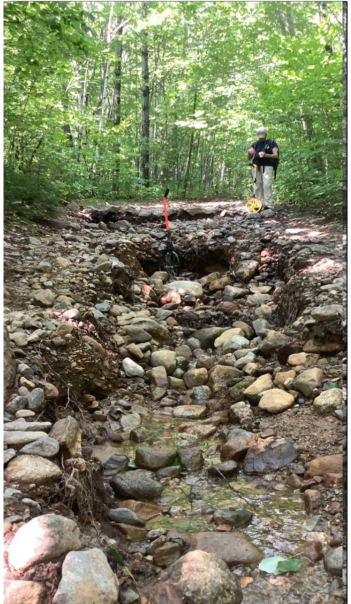
A section of the lower Brook Trail that was washed out after the 2023 storms
