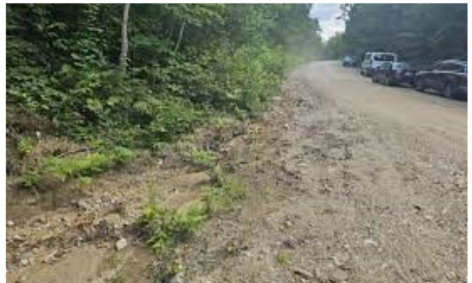
A washout on Byron Road, June 2023.
